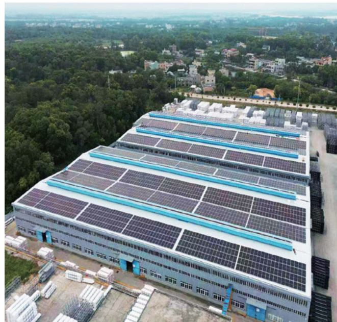
Dingan Roof Solar Power Station
