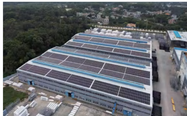
Dingan Roof Solar Power Station
