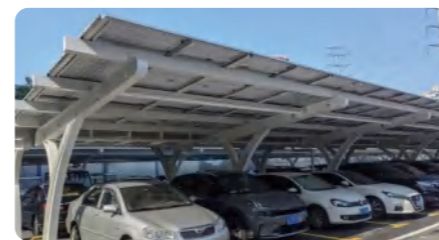
Waterproof PV carport
