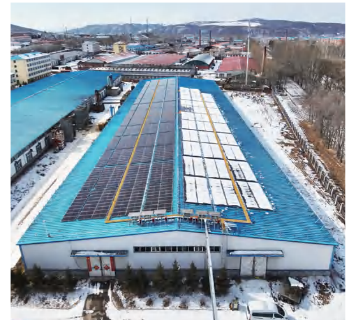
Mulingke Kemian Factory Roof Solar Power Station
