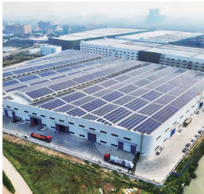
Haitian Roof Solar Power Station
