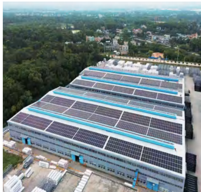
Dingan Roof Solar Power Station
