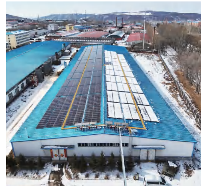
Mulingke Kemian Factory Roof Solar Power Station
